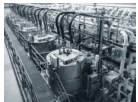
Installation with 42 gypsum centrifuges
