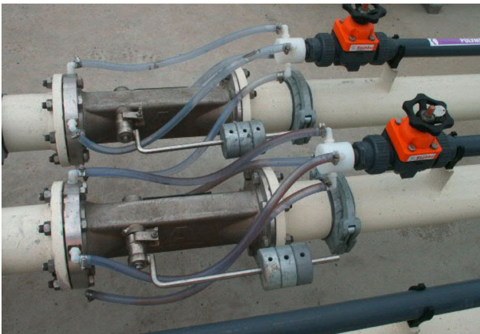
▲ Venturi mixer, inline flocculation system
